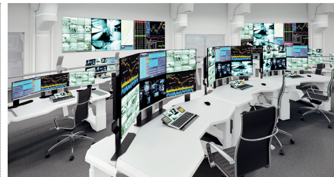
Wey, Control Room
